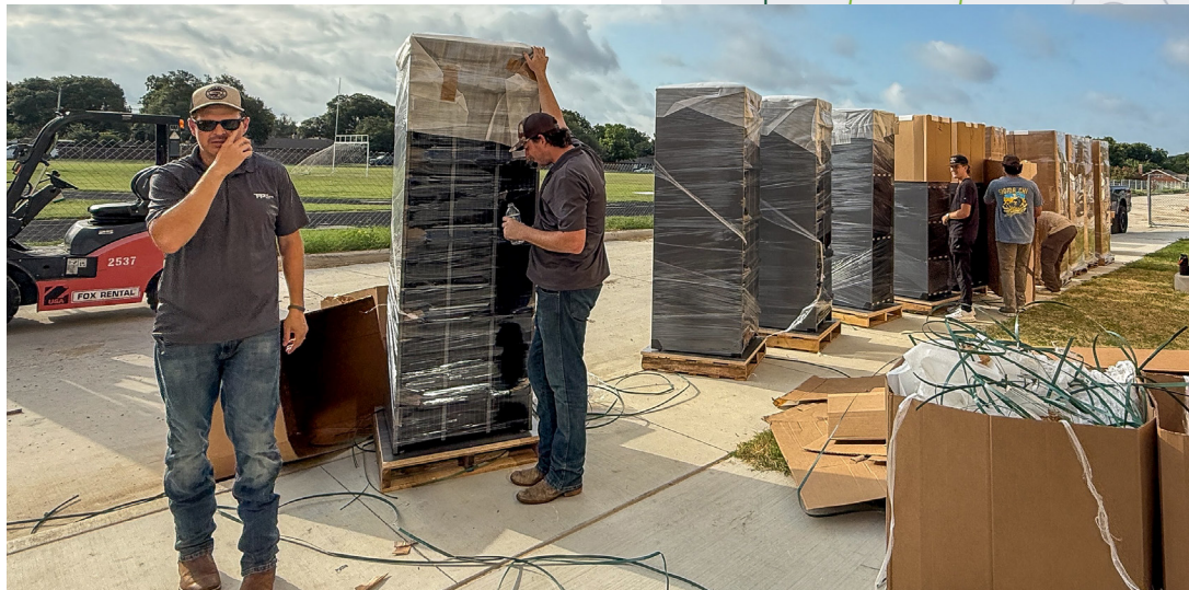
Installation-ready cabinets arrived fully assembled and protected.
